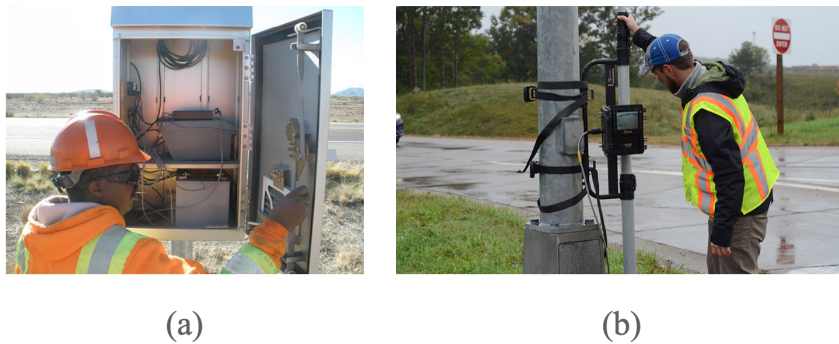
Figure 32: Installation of traffic stations by (a) Arizona DOT, (b) Wisconsin DOT.
